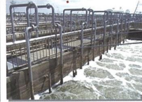
Temporary wastewater treatment facility (biological contact oxidation using a bio film method with string media.)
