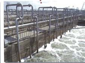
Temporary wastewater treatment facility (biological contact oxidation using a bio film method with string media)
